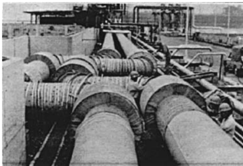
Figure 4.15 LNG Pipe Lines Insulated by Frothing-in-Place [4.54].
